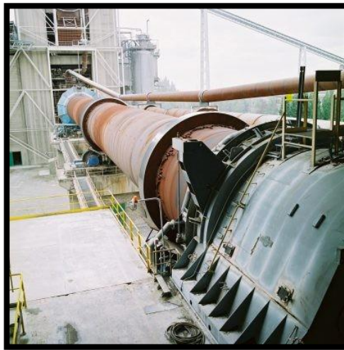
Figure04: Rotary cement kiln [48].
