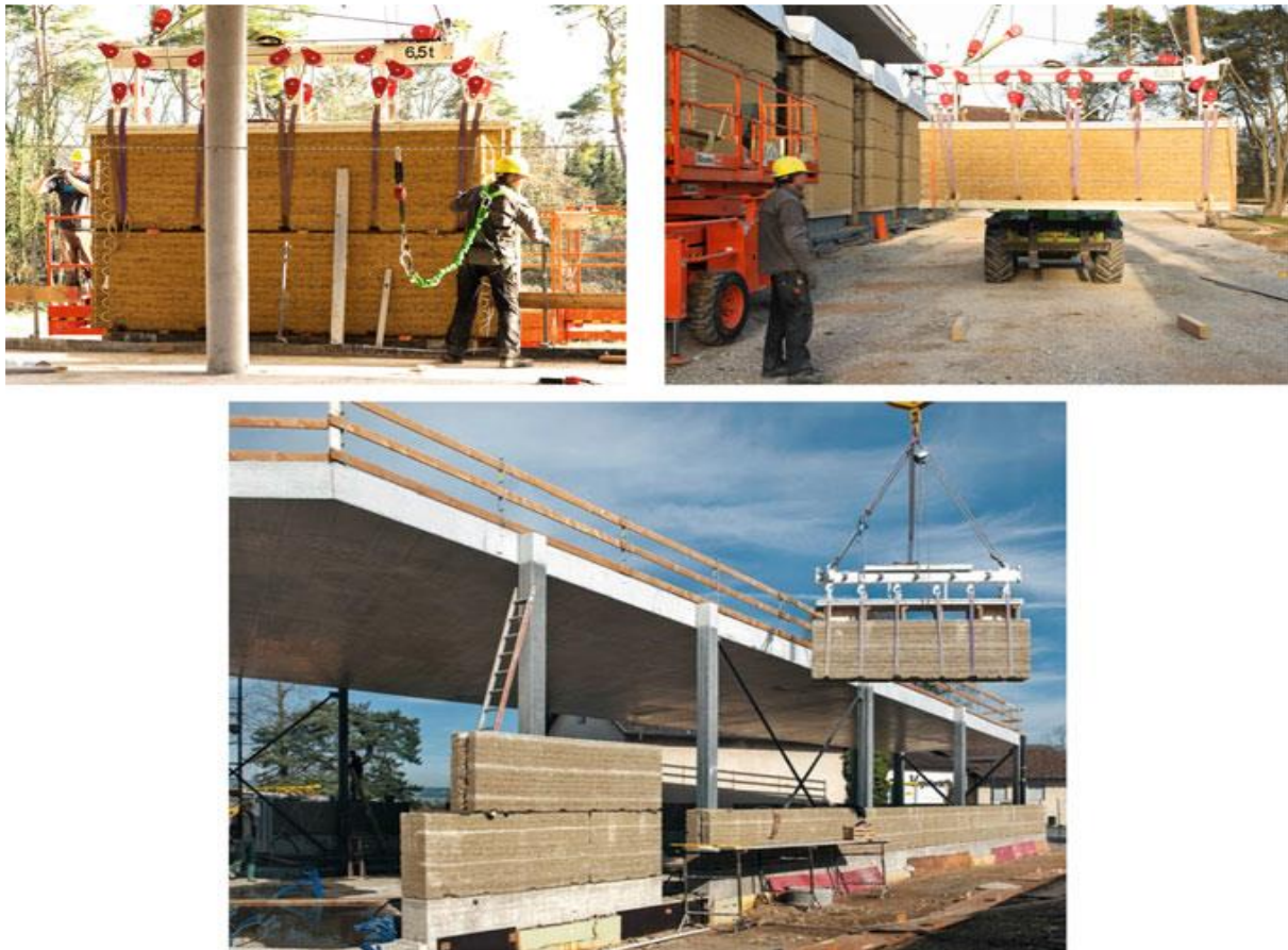
Figure 2.11 Unstabilised prefabricated rammed earth panels transported and assembled at site (Venkataram Reddy, 2022)
