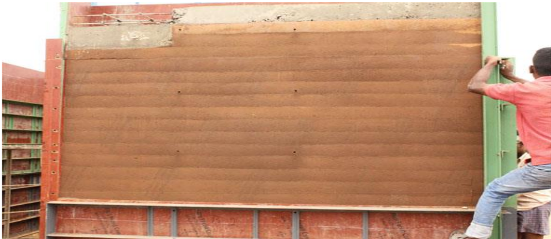
Figure 2.16 Part of the RE wall exposed during formwork stripping (Venkatarama Reddy, 2022)
