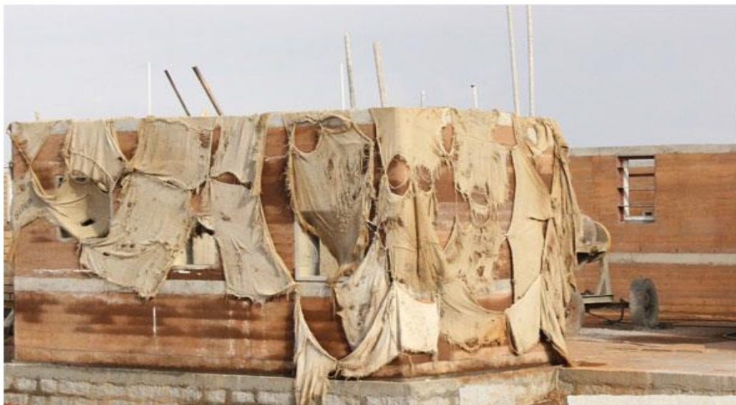
Figure 2.17 Cement stabilised rammed earth wall covered with burlap for curing (Venkatarama Reddy, 2022)
