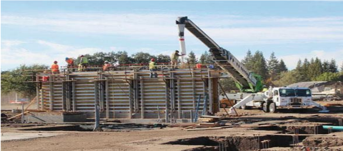
Figure 2.14 Formwork for the entire height and length of rammed earth wall (Venkatarama Reddy, 2022)
