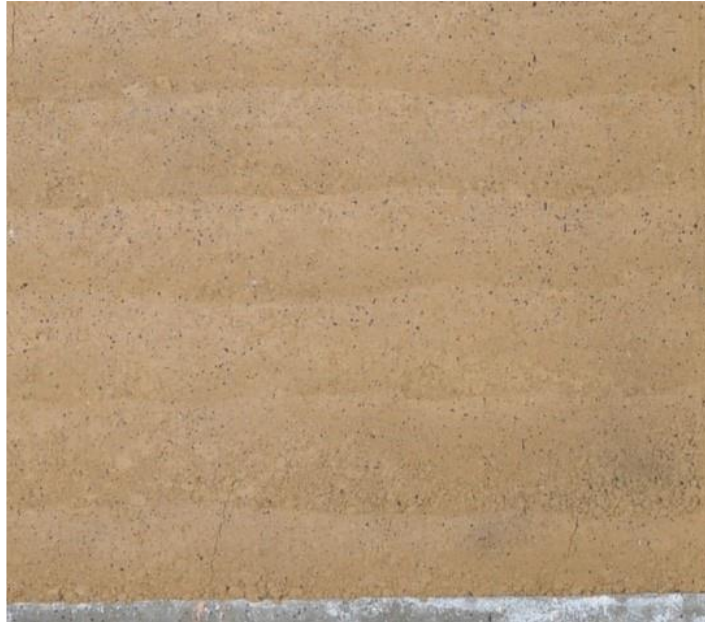
Figure 1.15 Visible compacted layers with different thickness of a rammed earth wall (El Nabouch, 2017)
