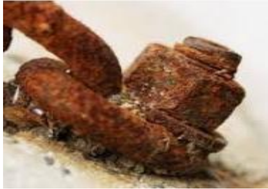
Figure I.3 La corrosion uniforme
