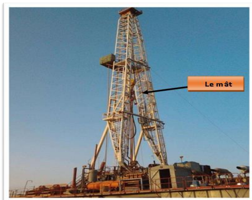
Figure II.8.Le mât de forage. [18]
