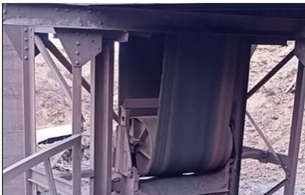
Figure IV.14 : Contrepoids [prise de la photo]
