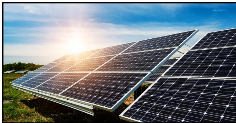
Figure 21: Panneaux photovoltaïques, Source : Boughriet, 2019.
