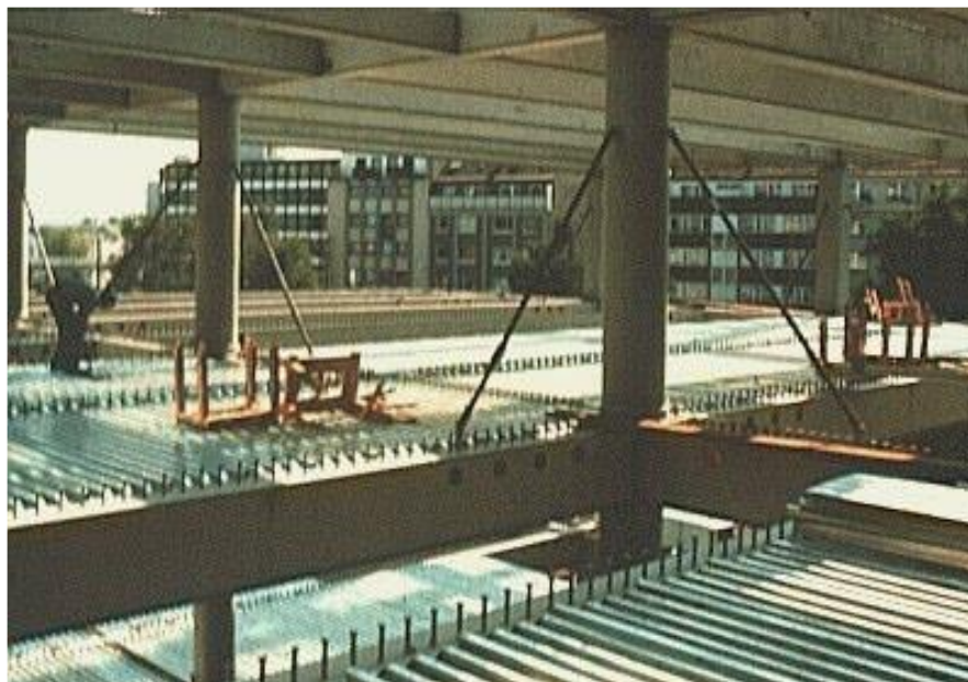
Figure 1. 6: The Usual Practice for Commercial and Industrial Buildings Is to Construct the Floors Using Metal Decking Which Is Embossed to Provide Composite Action.
