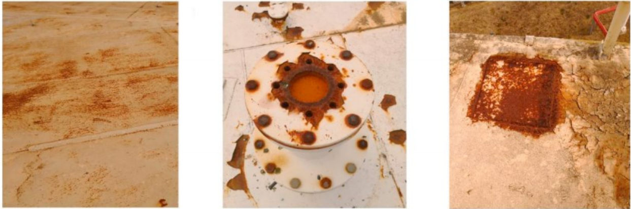
Figure 1.2 Example of damages in elements of the tank
