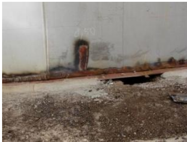
Figure 1.1 Bottom damage of a tank
