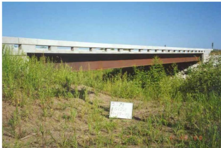
Figure2. 9snyder bridge south in nebraska. source: (azizinamini, van ooyen, jabar, & fallaha, 2002). reproduced with kind permission of prof. a. azizinamini.
