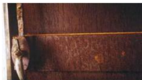
Figure- I .1 Corrosion uniforme
