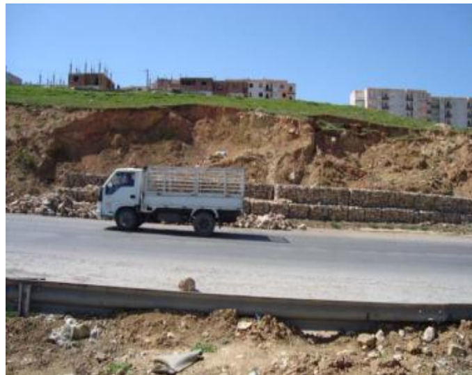
Figure 4.9 An example of a landslide where the slope fails due to scouring.
