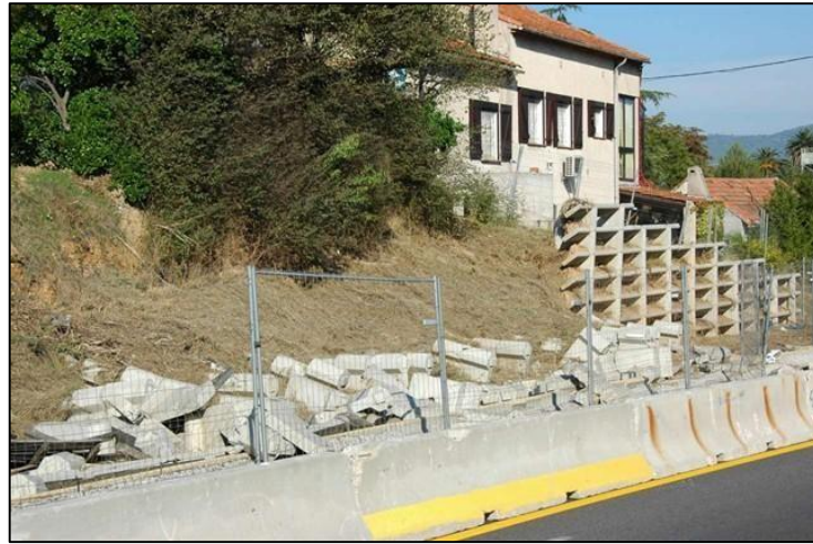
Figure I.31: Retaining wall of the RD559 in the Var, collapsed under the push of the slide, image A.Woimant
