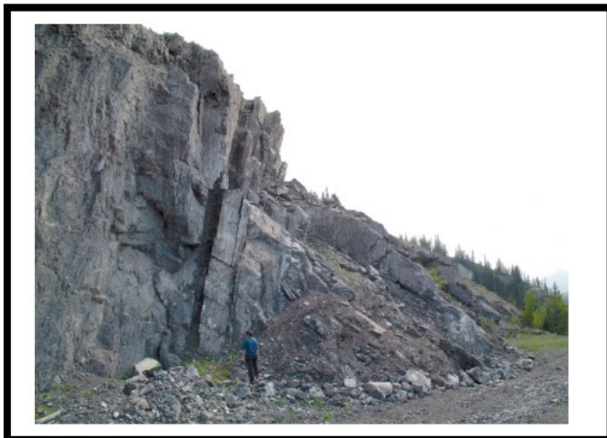
Figure 5: Photograph of block toppling at Fort St. John, British Columbia, Canada. (Photograph by G. Bianchi Fasani.)
