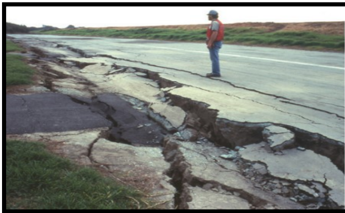
Figure 11: Photograph of lateral spread damage to a roadway as a result of the 1989 Loma Prieta, California,USA, earthquake. (Photograph by Steve Ellen, U.S. Geological Survey.)
