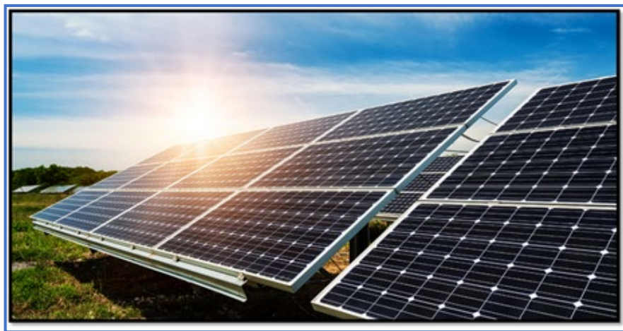
Figure 1.14 1: Panneaux photovoltaïques. Source : Chahinez,2021.
