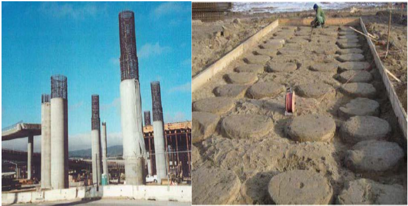
Figure 2.12 Foundation support executed by SM method. a) Railroad Bridge supported by deep mixing column at San Francisco International Airport (Porbaha, et al., 2005), b) columns under the foundation for A2 Motorway near Katowice, Poland (Massarsch & Topolnicki, 2005) [17]
