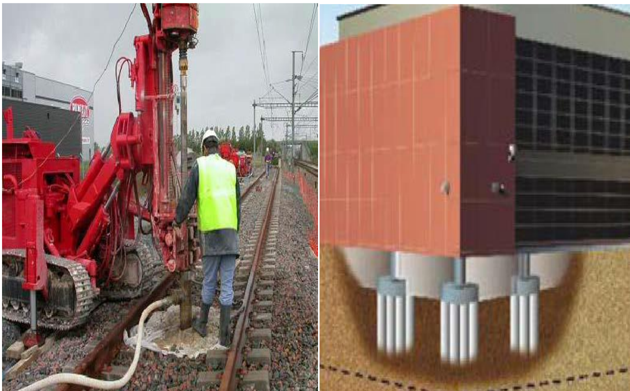
Figure 2.13 Application of SM: a) under the railway track (INNOTRACK, 2009), b) under building foundation (Nozu, 2005)
