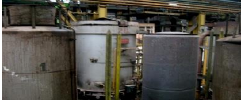
Figure III.6. Bassin de recuit
