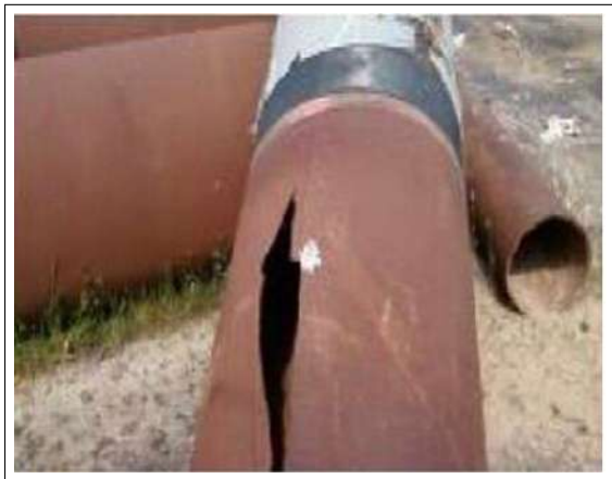
FIGURE 2.7 – Rupture d'un pipeline [19]
